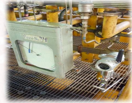
Automation of taking of readings of Pressure in different points Installation.
